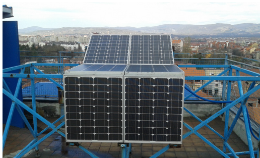
Fig. 1. Monocrystalline silicon solar modules ISF-60/12 on the roof of the Faculty of Sciences and Mathematics in Nis, used in the experiment
