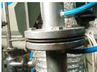
Fig. 3. Orifice connection on the line
