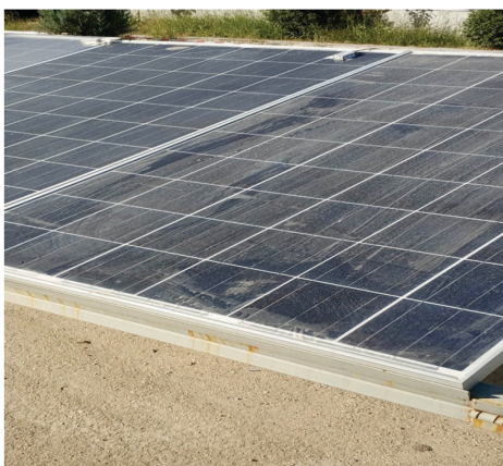
Fig. 2. Pollution formation on the uncleaned photovoltaic panel surface
