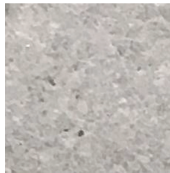
Fig. 1. Image with negative crack detection
