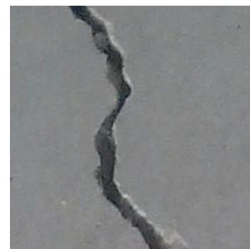
Fig. 2. Image with positive crack detection
